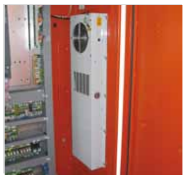
Built-In Heat Exchanger
