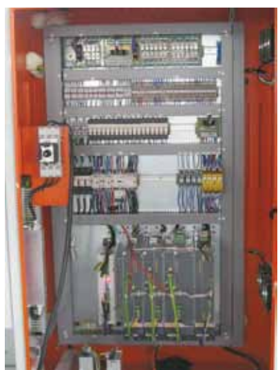
CE-Marked Electric Cabinet
